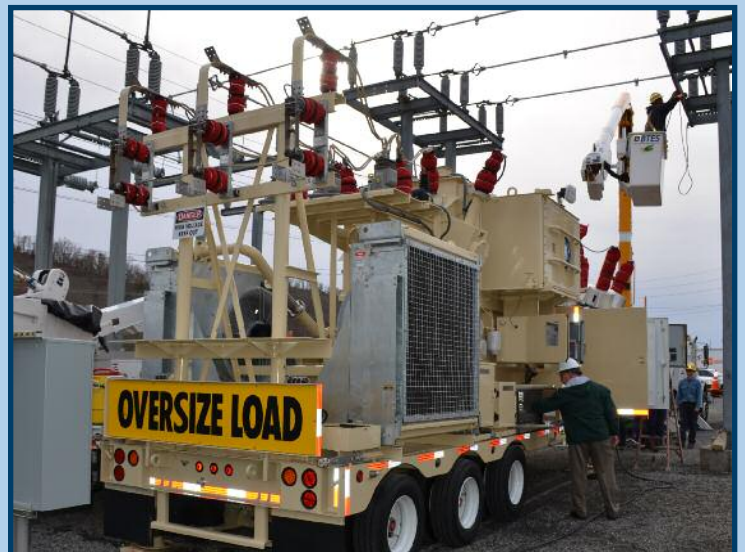
BTES’ mobile substation arrived in early December 2016. Crews immediately began training on its operation and capabilities.
